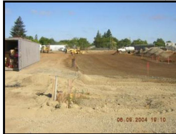
Elvas Avenue (St. Francis HS) – LFG Control System
